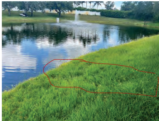
Erosion on east side of the lake; Approximate 6 inch drop This area is not safe
