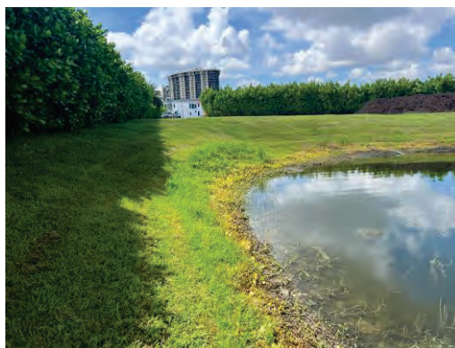
Slope appears to be greater than 4 to 1 on south side of lake This area is not safe
