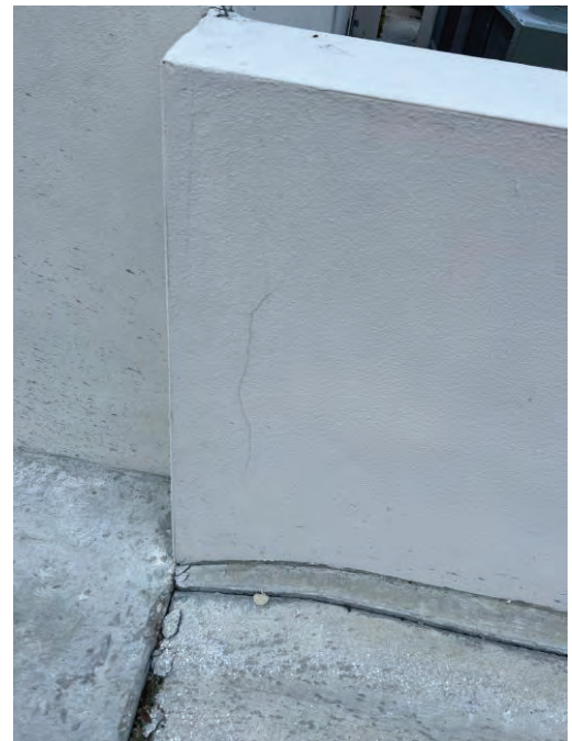
Damaged concrete wall in the proposed parking garage (typical)
