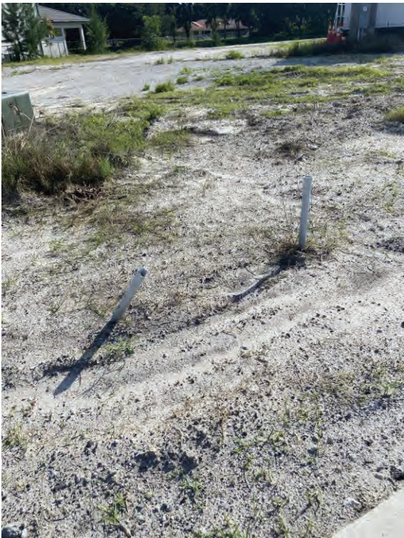
Sharpe edged standing pipes on the side of Baneberry Ln
