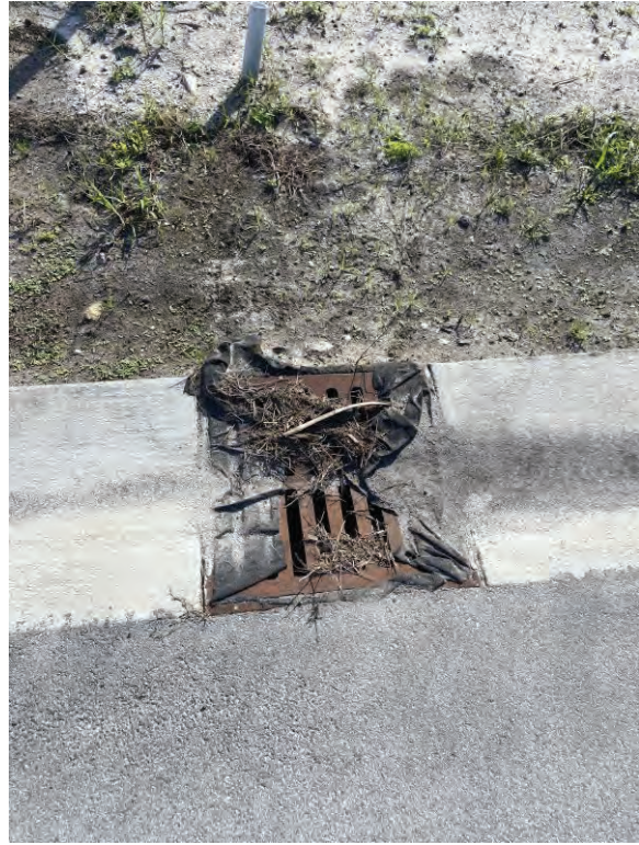
Catch Basin clogged by debris; filter fabric cover has been ruptured and is now opened (typical)
