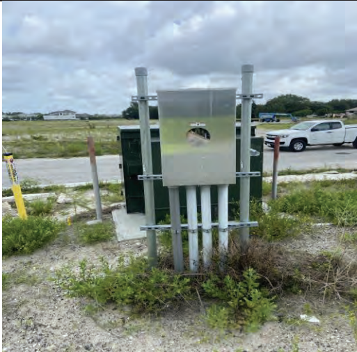
Uncovered electric box
