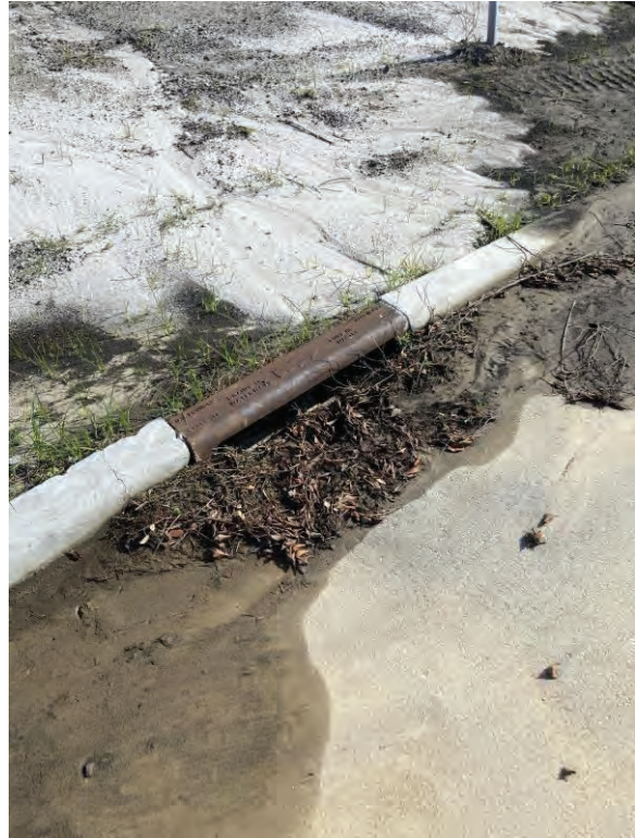
Stormwater inlet clogged by debris
