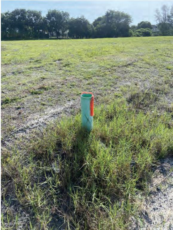
Cleanout with no cover/cap (typical)
