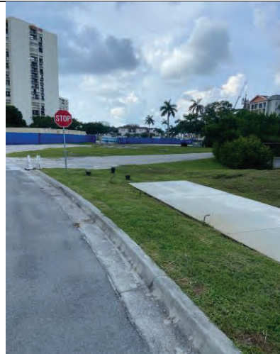
Unfinished Sidewalk on the SW side of the Banyan Club Rd
