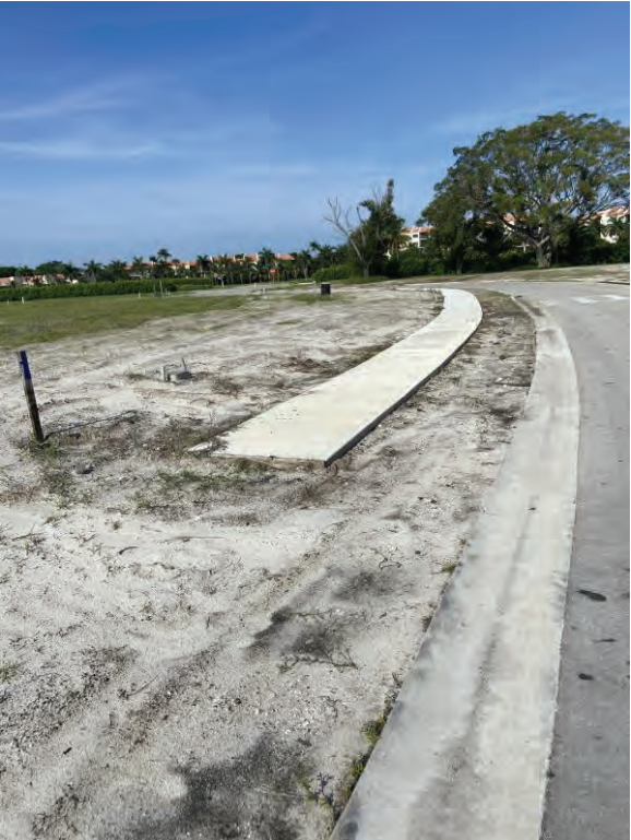
Unfinished sidewalk on Baneberry Ln
