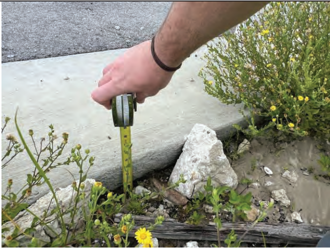
Valley gutter curb damaged due to erosion
