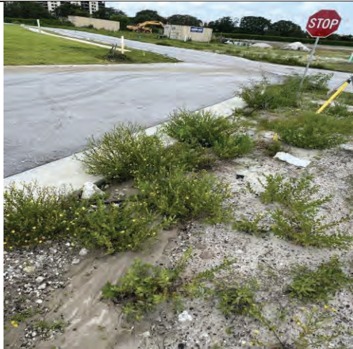
Overgrown valley gutter curb
