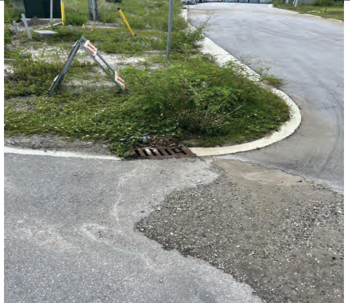
Banyan Resort Way – Overgrown Catch Basin
