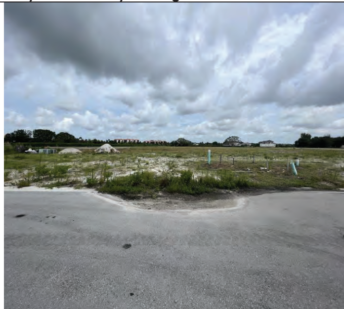
Banyan Villa Circle – Overgrown valley gutter curb
