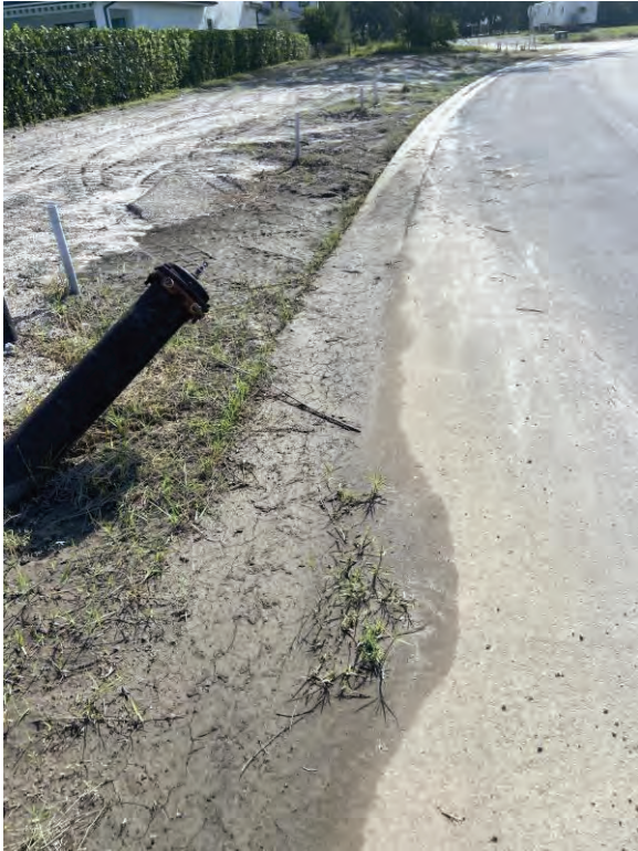
Valley gutter curb filled with dirt
