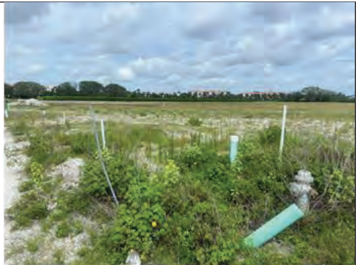
Cleanout missing cover/cap
