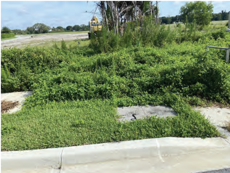
Unfinished sidewalk on Banyan Resort Way
