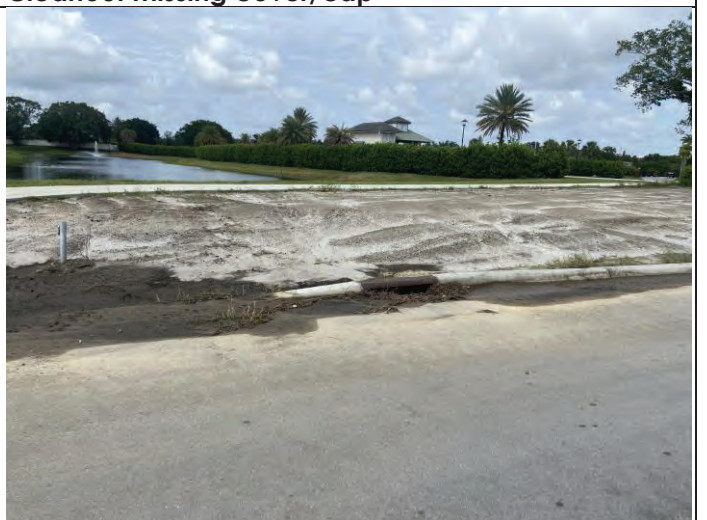
Baneberry Ln – Valley gutter curb filled with dirt
