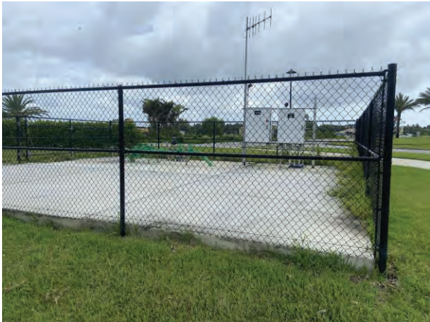
Lift Station West of the Banyan Club Rd
