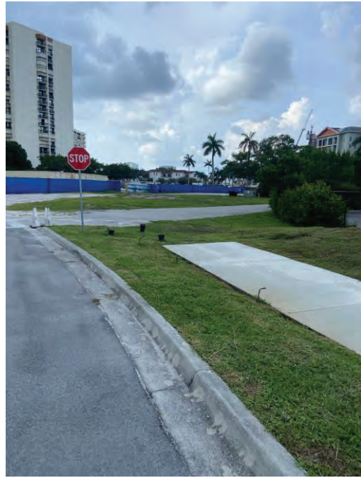
Unfinished Sidewalk on the SW side of the Banyan Club Rd
