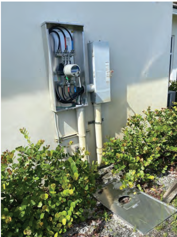
Opened electrical box on the N side of the Fitness Center
