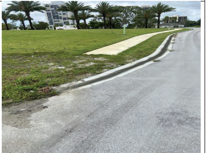
Banyan Resort Way – Unfinished sidewalk
