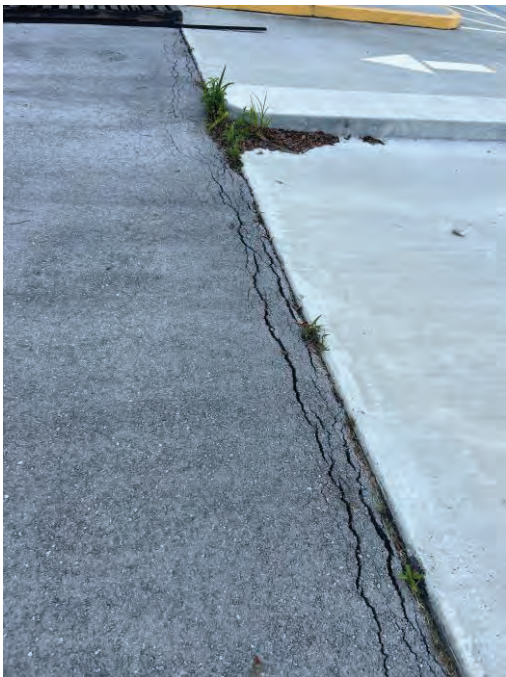
Damaged asphalt in the proposed parking garage
