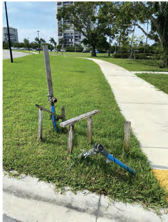
Eagle Oaks Ln SE end: Unstable Backflow Preventer
