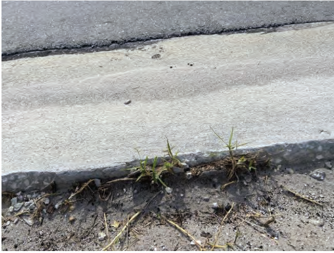
Valley Gutter Curb damaged due to erosion
