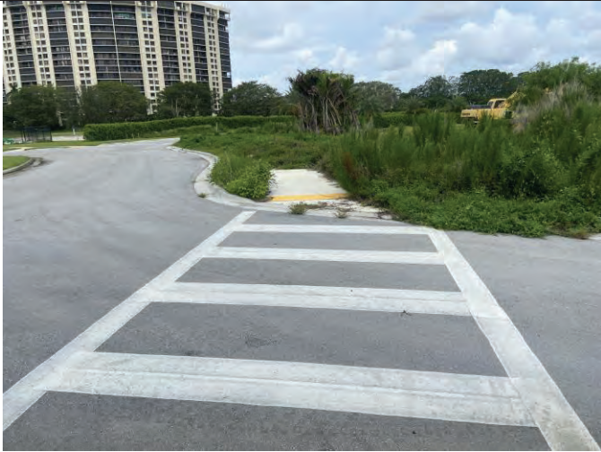
Banyan Resort Way – Overgrown sidewalk
