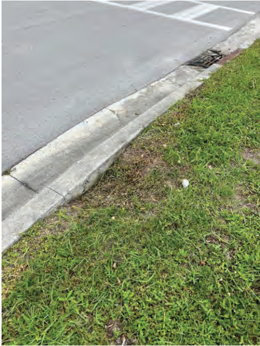
Curb damaged due to erosion – Banyan Club Rd
