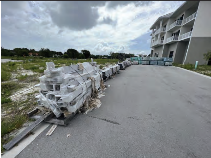
Unused material stored on the NE side of the hotel
