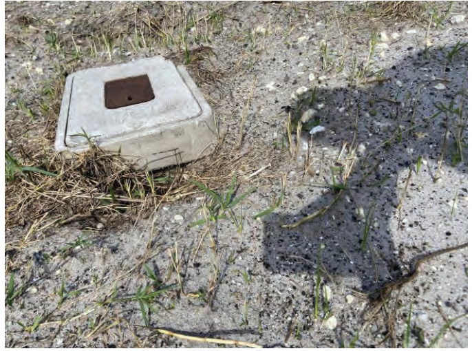
Water Meter damaged due to erosion
