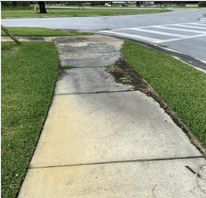
Banyan Villa Circle – Damaged sidewalk
