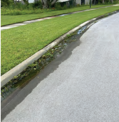
Banyan Club Rd – Overgrown side curb
